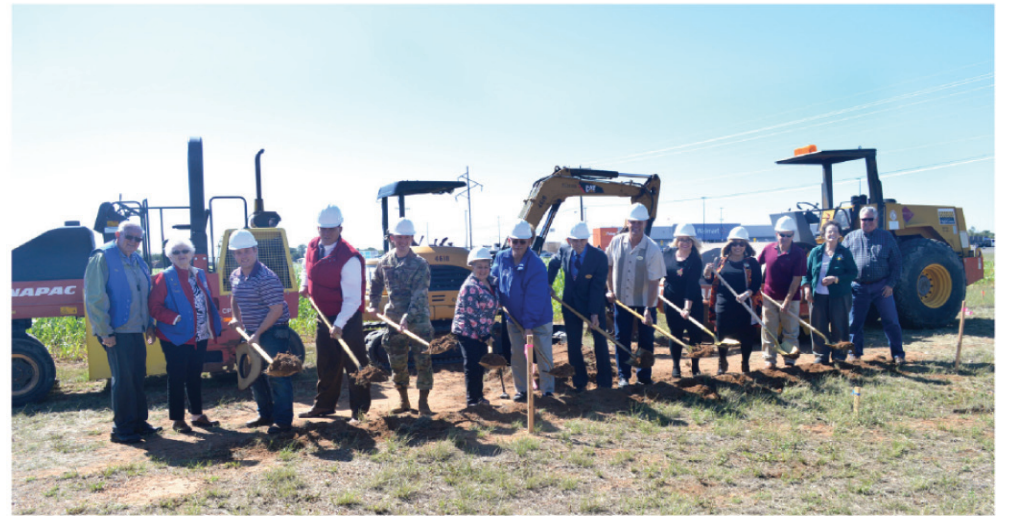
The officers and board of Cannon Federal Credit Union officially broke ground on the organization's new location in Portales in October. The Kilgore Avenue and Spruce Street location will be home to a drive-thru ATM location within 90 days and a full branch location is anticipated in the future according to President/CEO Heather Fowler. Fowler added that any resident of Roosevelt County is eligible for membership in the credit union. Members of the Chamber, Ambassadors and Roosevelt County Community Development Corp. were on hand to help with the ceremony.
